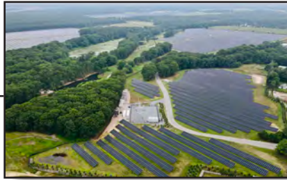
Calverton Solar Energy Center (22.9 MW) Calverton, New York
