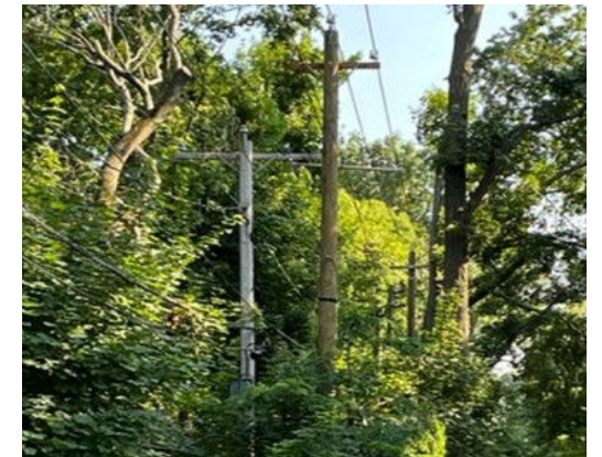
Figure 4. Improved circuit included in the Power On program prior to removal of original poles.
