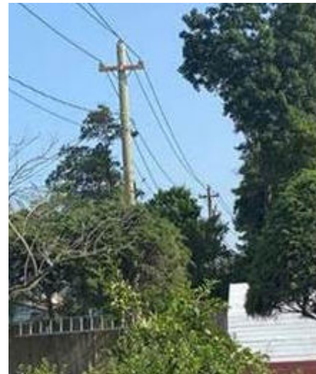
Figure 2. A storm-hardened distribution circuit.
