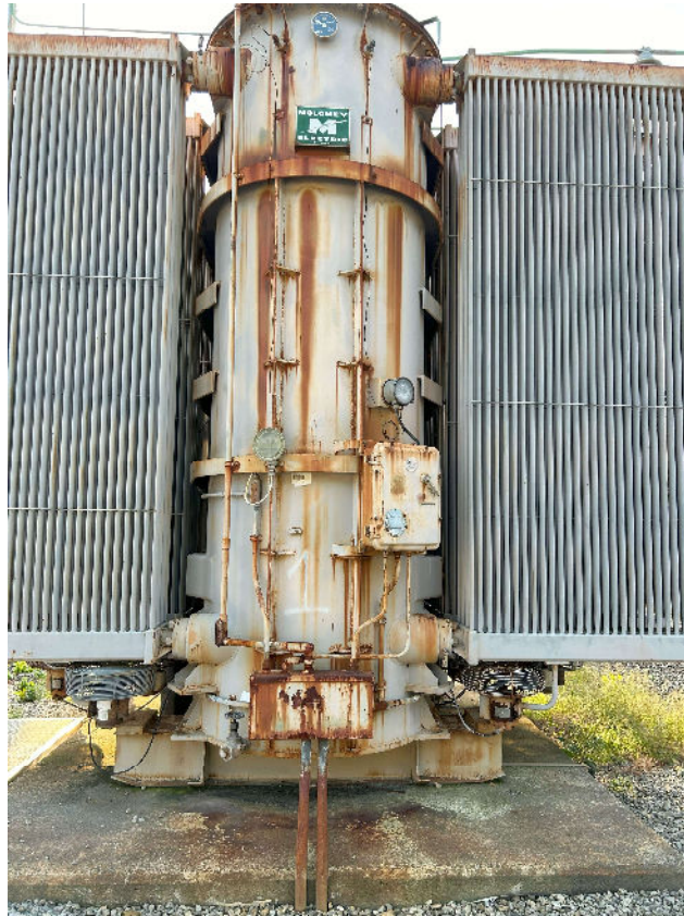
Figure 4-2: Moloney Transformer in Eastport Substation
