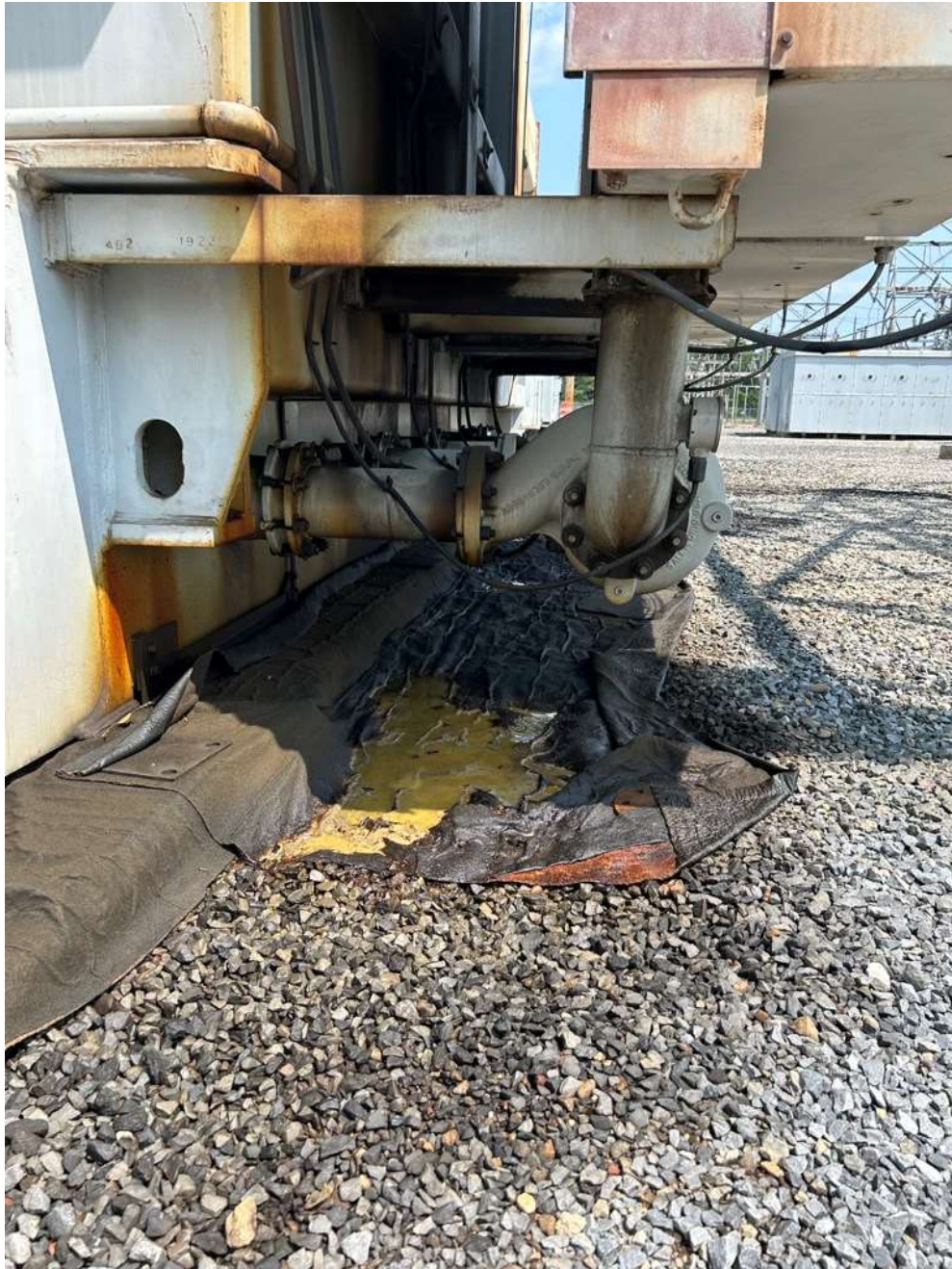
Figure 4-7: Signs of a Transformer Oil Leak at Ruland Substation
