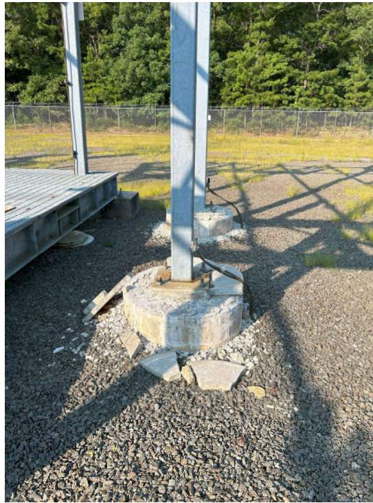
Figure 4-1: Pile Cap Deterioration
