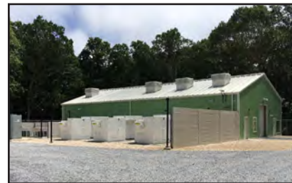
East Hampton Energy Storage Center (5 MW) East Hampton, New York
